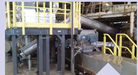
Completed Ineos Salt plant upgrade
